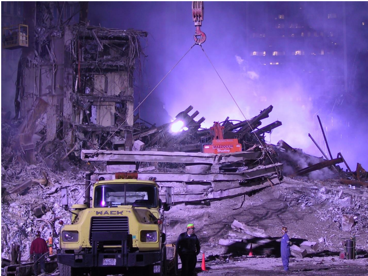
Figure 24: Wall boards surround the stairway where 13 survivors of the North Tower demolition were located suggesting horizontal propellant forces were absent at this location and falling debris did not dislodge wall board material.
